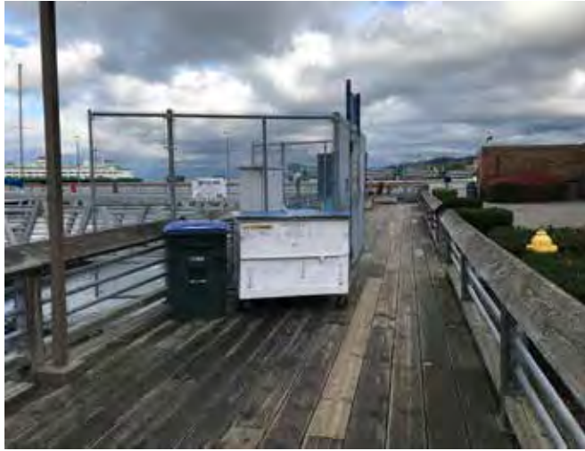
Security gates cause impingement on pedestrian clear space, leading the marina to not meet current ADA standards
