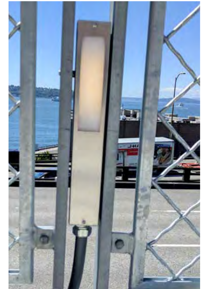
Fixture showing housing and translucent fixture lens to diffuse and reduce potential glare issues
